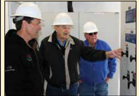
CMS Manager Kirk Thompson (left) and Board member Don Nighswonger (right) watch as former Board member Darrol Miller energizes the substation.
