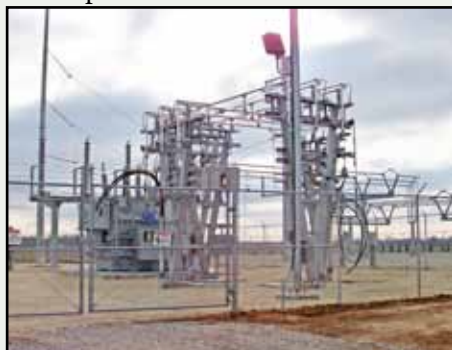
The Maize Substation was energized last month.
